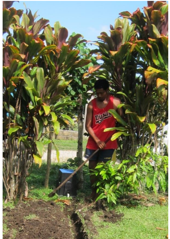
Figure2. Akosita Rakisiica's son from Ha'atafu digging a new trench to connect their home to the new village water supply water meter
