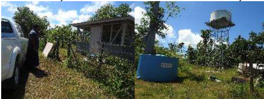
Figure 22: Flow meter installation
