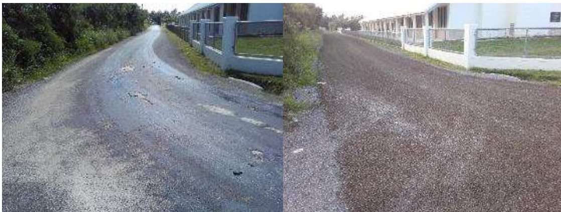
Figure 12: Popua Evac. Road 15 Oct. (left) bleed caused by heavy machineries. Repaired 2nd Nov. 2018 (right).
