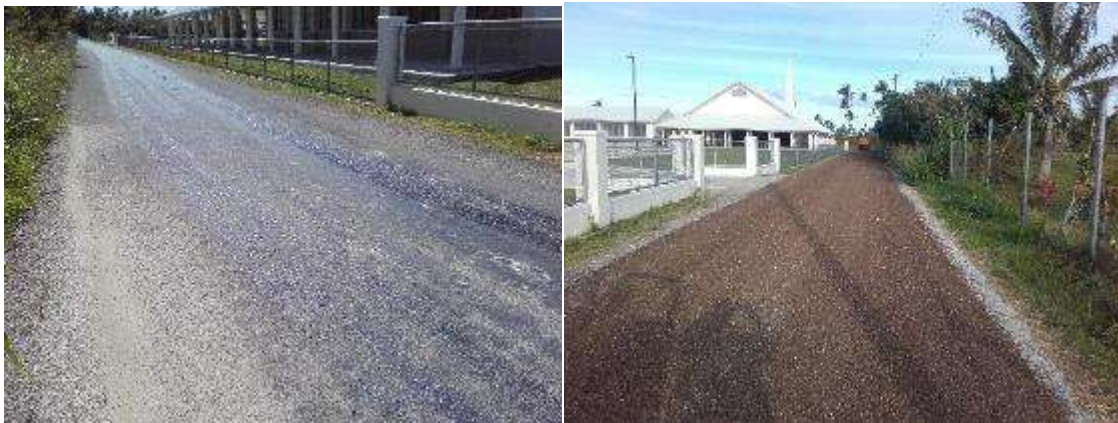
Figure 11: Popua Evac. Road 15 Oct. (left) bleed caused by heavy machineries. Repaired 2nd Nov. 2018 (right).
