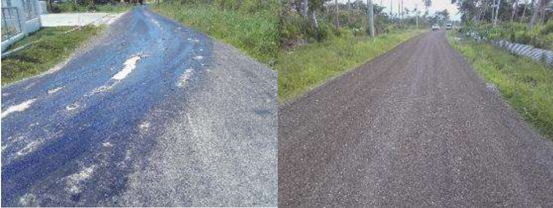
Figure 13: Popua Evac. Road 15 Oct. (left) bleed caused by heavy machineries. Repaired 2nd Nov. 2018 (right).
